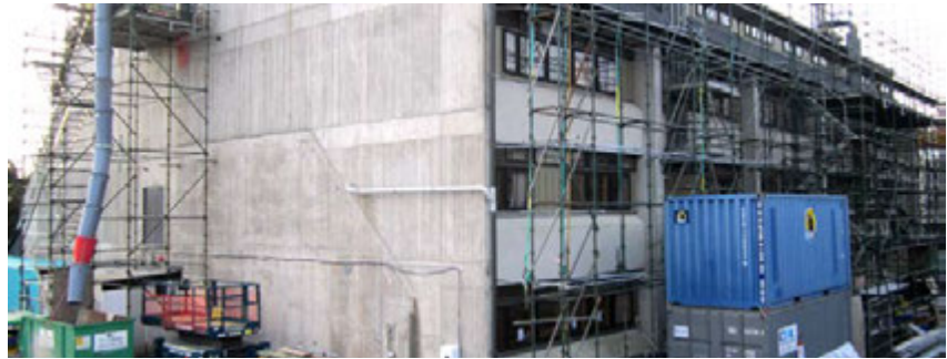
Repairs to quake damaged Christchurch Girls' High School were carried out while the school was still open.
