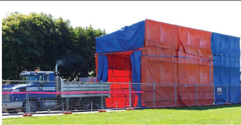
The mother of all car washes: spotted at Westland High School. Trucks getting washed as a precaution after removing fire damaged material from the school before staff and students returned.
